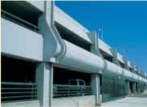
Large bullnose components added to the parking structure at the Hyperion Wastewater Treatment Facility provided a distinctive visual element that tied it to the other buildings in the project without mimicking their exact look.
